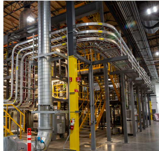
Pilot plant of a molten chloride reactor of the company TerraPower (Source: TerraPower)
